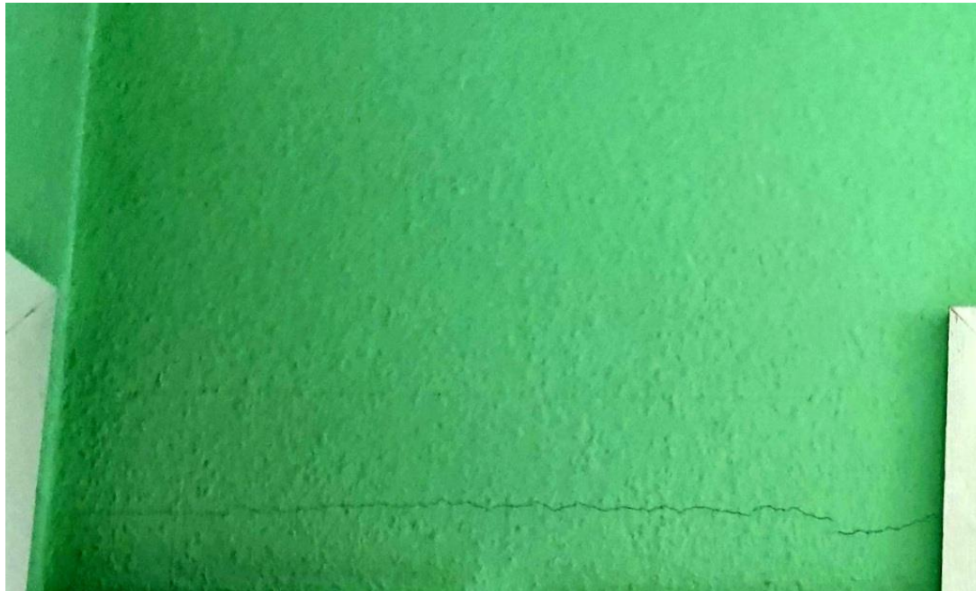
horizontaler Riss in Innenwand
